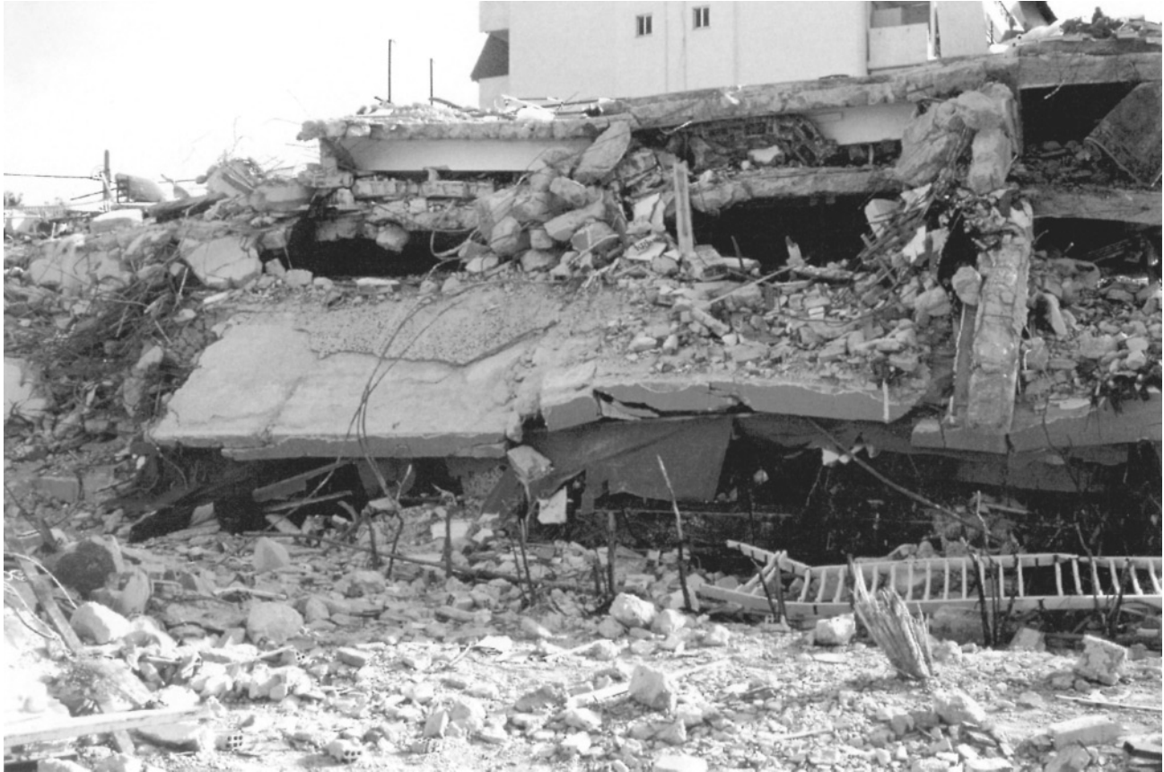
Figure 1. A typical example of structural damage (column failure followed by collapse) of a three-story residential reinforced-concrete building at about 8 km from the epicenter on soft soil.
